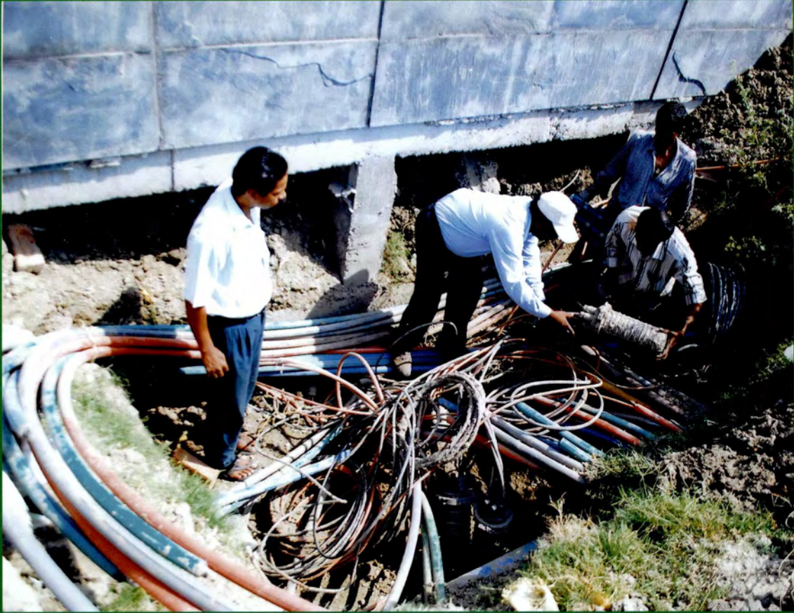
Laying of Telecom Infrastructure (Underground duct) in progress in New Town by NTTIDCO Ltd.— a Subsidiary Company
